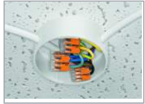
Lighting distribution in a ceiling canopy
